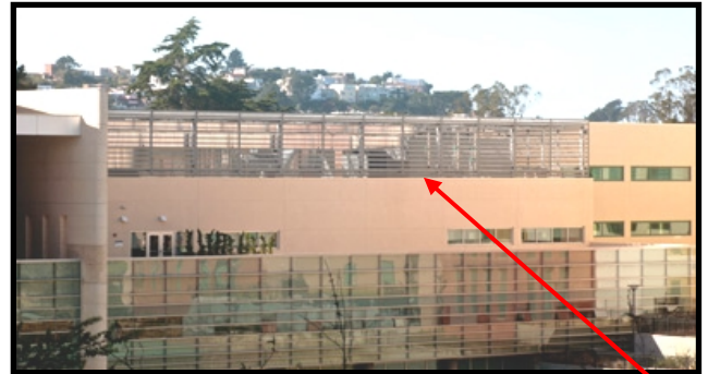
Generators and air handling equipment were installed on the roof of the new hospital.
